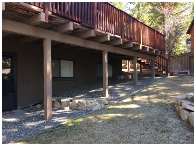
Figure 5: The under-deck area should be considered in the noncombustible zone, including managed vegetation and removing combustible materials. (Photo: Shearman Builders)
